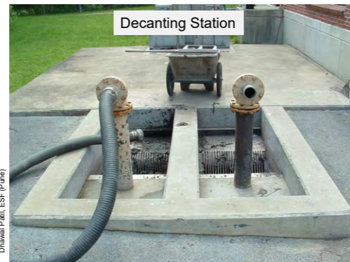
No splashing / spillage during decanting
