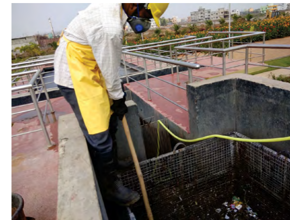
Screen basket without adequate access
