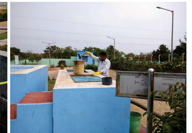
Enclosed screen with potential hazard of gases
